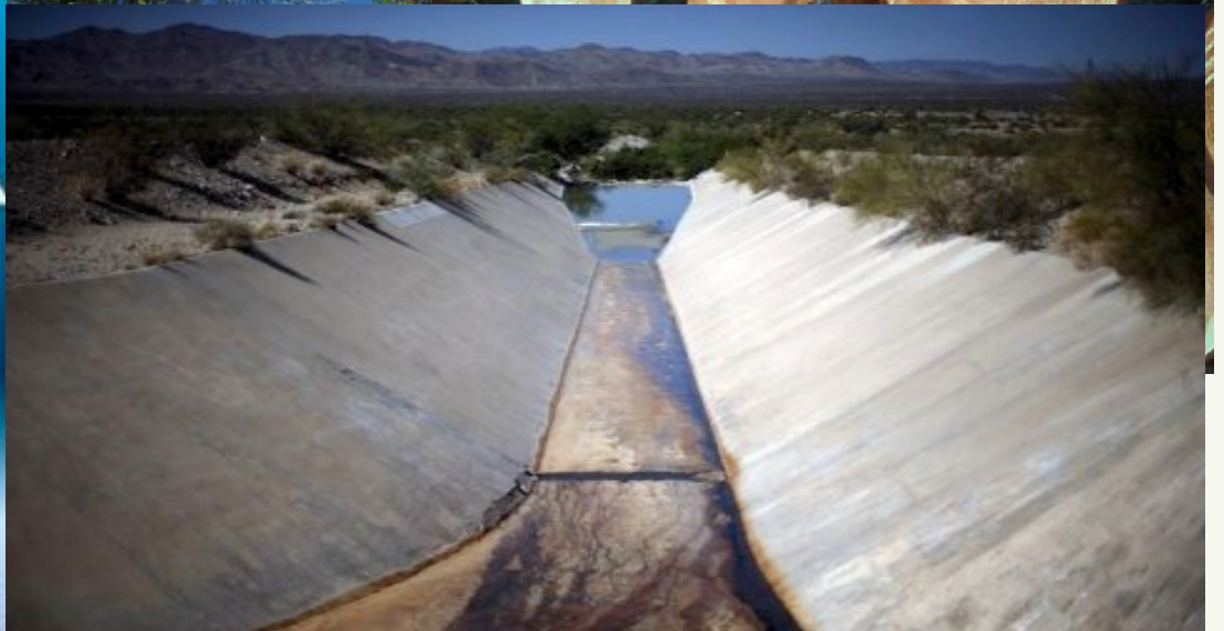
Colorado River aqueduct, ,California (Reuters)
